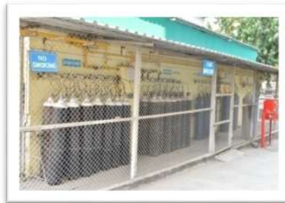
CYLINDER MANIFOLD ( Tertiary )
